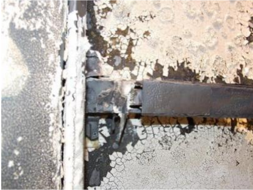
Exposed door face after the termination of the test – lock.
